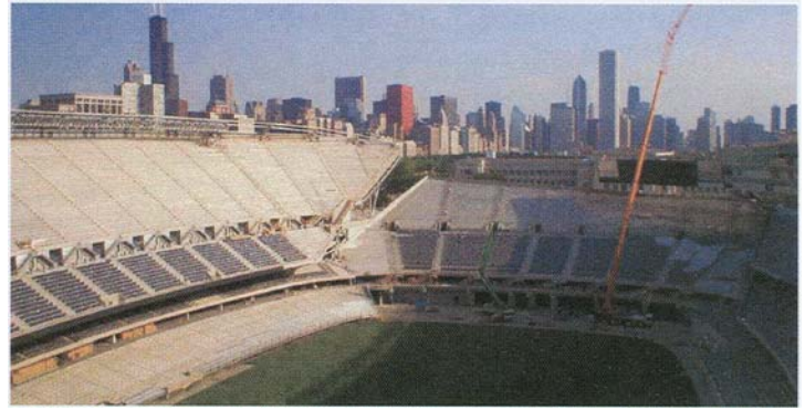
Pipe supplied by Can Clay Corp. for the renovation at Soldier Field.
